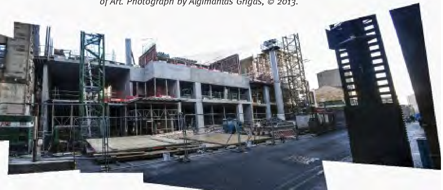
Building work progresses at the Glasgow School of Art. Photograph by Algimantas Grigas, © 2013.
