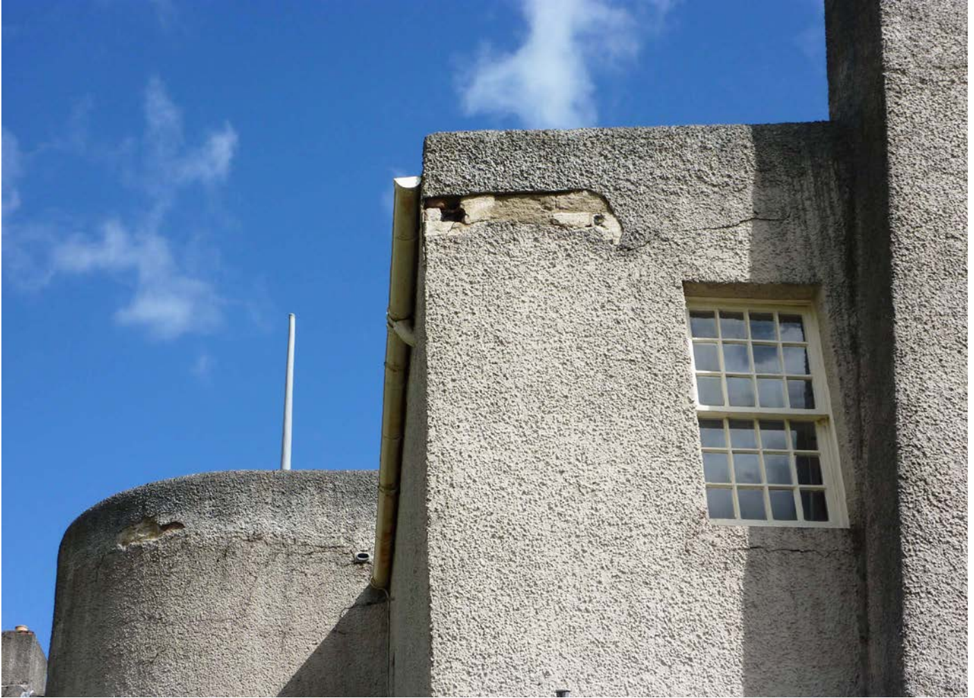
Harling decay at The Hill House
