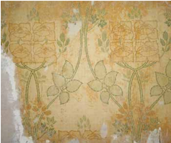
Fig. 14 A small section of original printed wallpaper surviving in the servant's quarters. Image: © John Cowie
