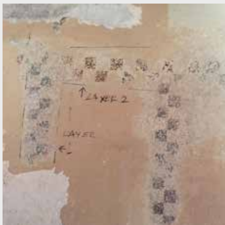
Fig. 5 The upper part of the wall in the dining room revealed an original stencilled scheme of repeating chequer-bordered squares and rectangles. This photograph of the dining room wall shows two different schemes of the chequer pattern applied at different periods.
