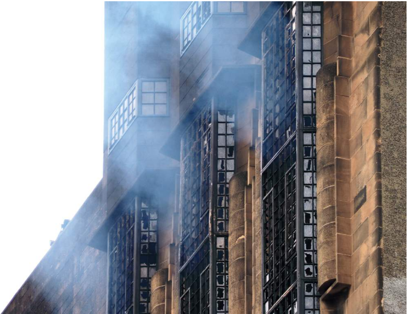
The day after the fire, smoke still smoulders from the Library of the Mackintosh Building © Stuart Robertson
